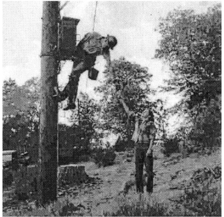
Reid (on pole) & Adele Marks working at the junction box between long-distance and local phone lines.
